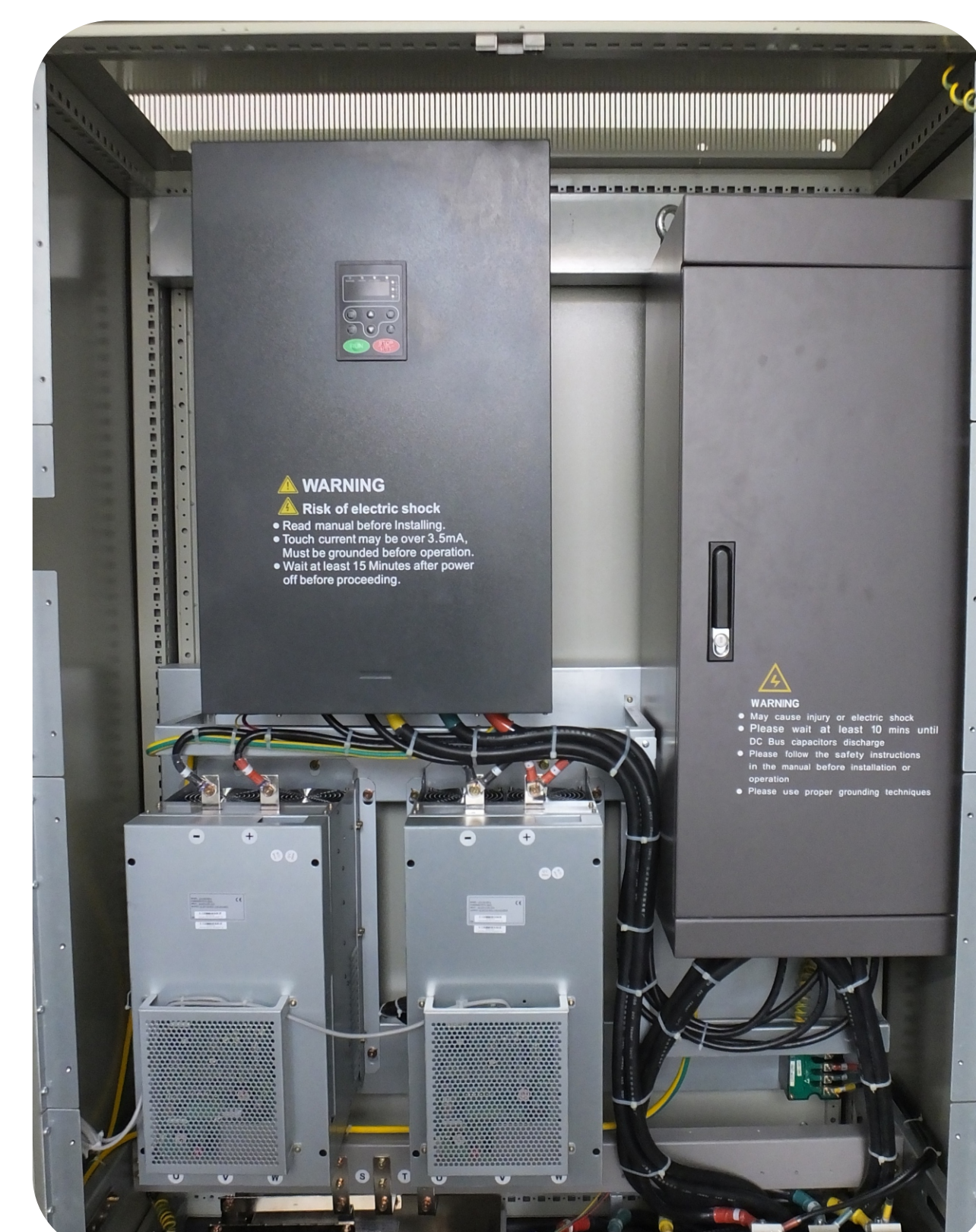
Motor Control Cabinet
